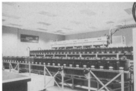
Fig. 1. Battery rack design.
